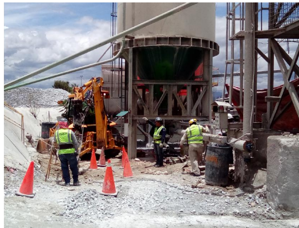
SILO CEMENTO MINA MARLIN, SAN MIGUEL IXTAHUCAN, SAN MARCOS, GUATEMALA
